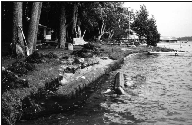
Figure 28: Coir staked in place, with sod excavation and stockpiling, and sand backfilling in progress.
