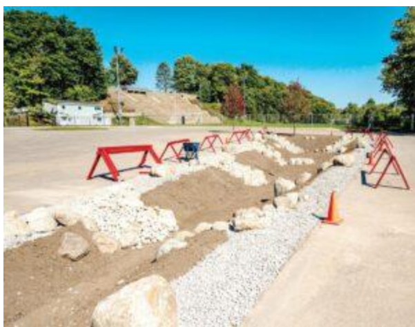
A rain garden is being installed at the Ottawa Stadium parking lot.
