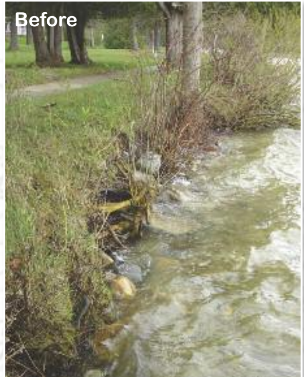
Exposed roots and undercutting along the Columbus Beach Club shoreline as indicators of moderate to severe erosion.
