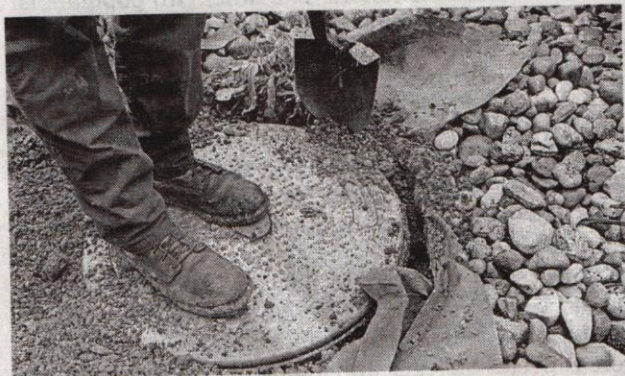
Brandon Eldridge, 29 of Charlotte, Mich. and a worker for Ball Septic, adds an extension to an already existing septic tank at a home in Lansing on Oct. 8. ERIC SEALS/DETROIT FREE PRESS
